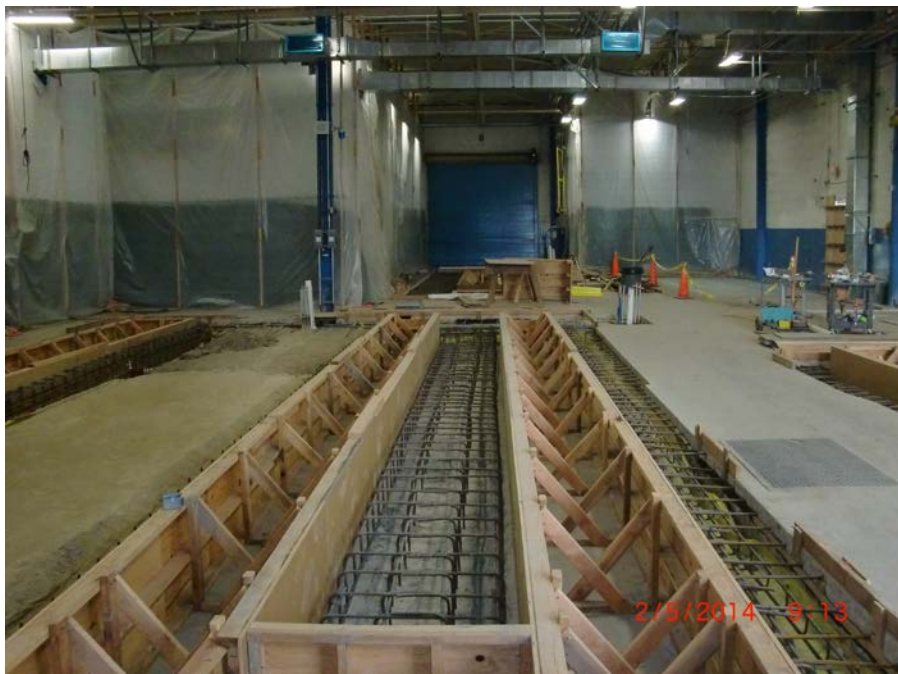
2. All 8 Underground Storage Tanks Are Removed, Buildings B and C are Demolished and Site is Being Prepared for Grading Activities and Foundations of Future Bus Wash and Fueling Stations
