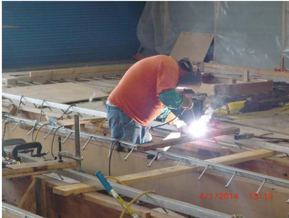
1. Installing Embed Angles for the New Bus Lifts in Building A (Maintenance Facility).
