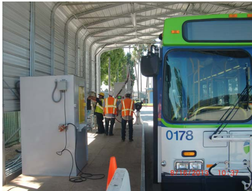
2. CIMG7828 = Testing of the Fleetwatch and GFI systems at the Temporary Fuel Island (Building D)
