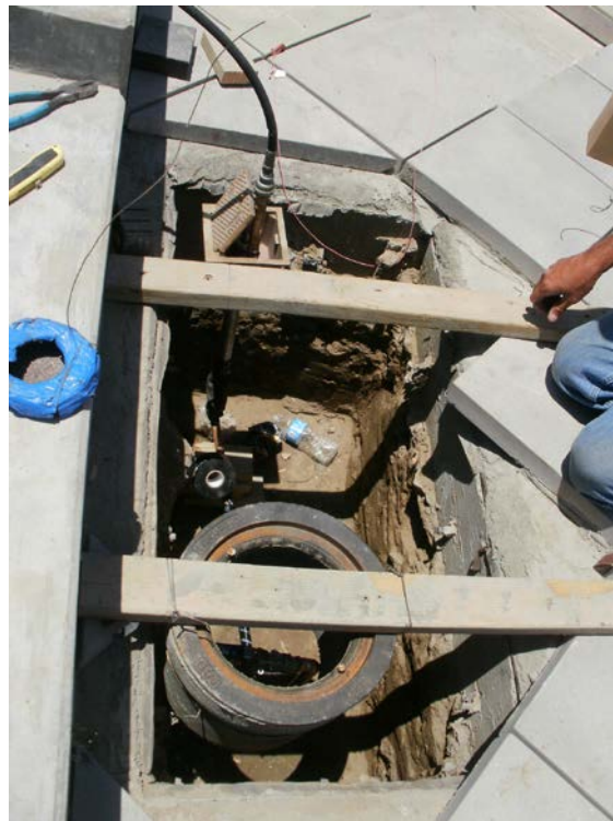
2. Connecting a hose bib to the potable water line at Highland Avenue and E Street.
