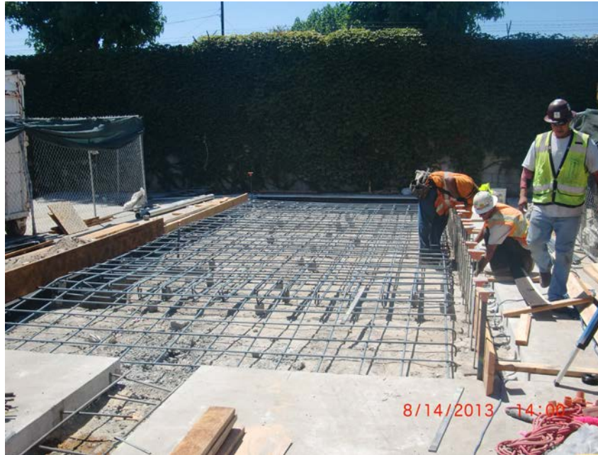
1. Reinforcing steel being set for the new trash compactor pad west of the Maintenance Facility (Building A)
